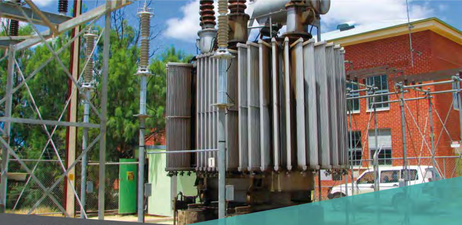
Morgan-Whyalla 2 Pump Station
